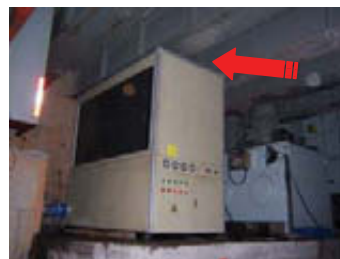
No air circulation clearance at airflow outlet
